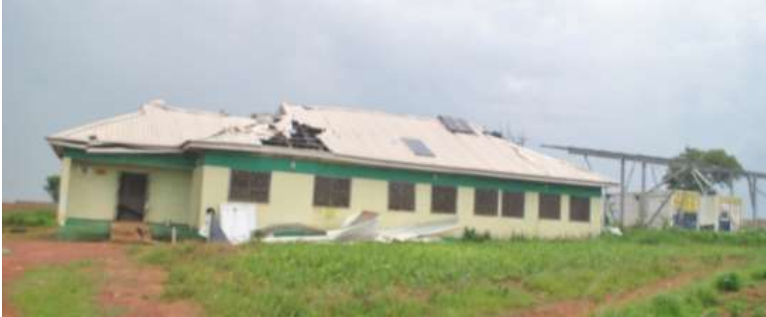
Image 5: A roof affected by wind.
