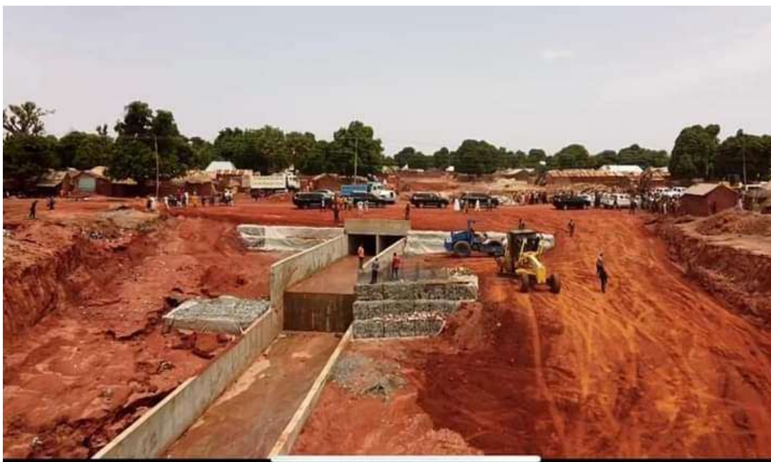
Plate III: Reclaiming of gully through proper construction of drainage channels in Rafin Gora
