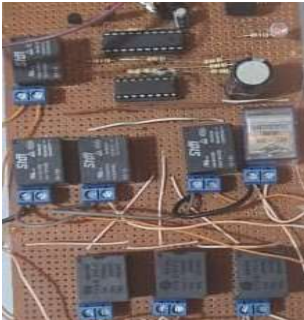
Figure 3a The SPDT circuit Board of the 8-channel relay
